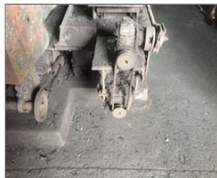
Photo of non-conformity NC of PA7.17.2.jpg
