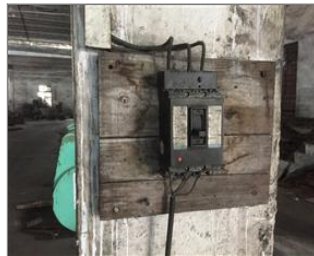
Photo of non-conformity NC of PA7.13.jpg
