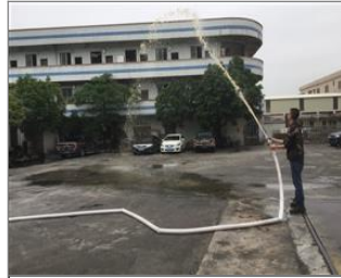
Photo of fire safety equipment Fire hydrant with testing.jpg
